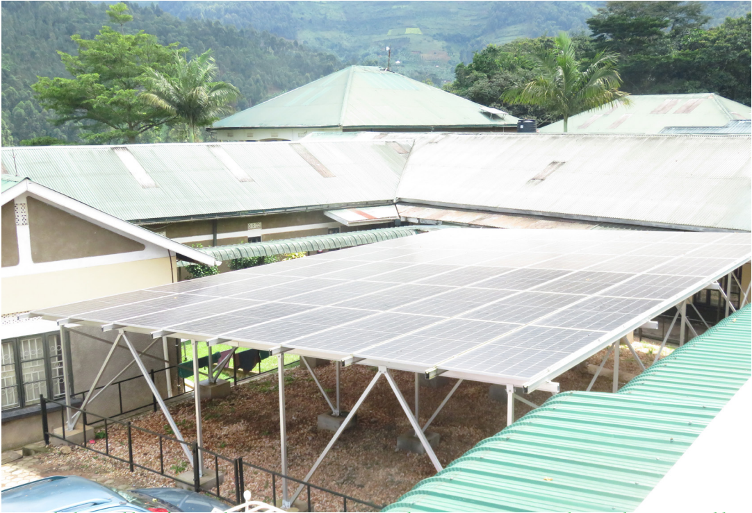
Solar panels donated by Africomed are now powering Bwindi Community Hospital, providing sustainable energy to support essential healthcare services.
