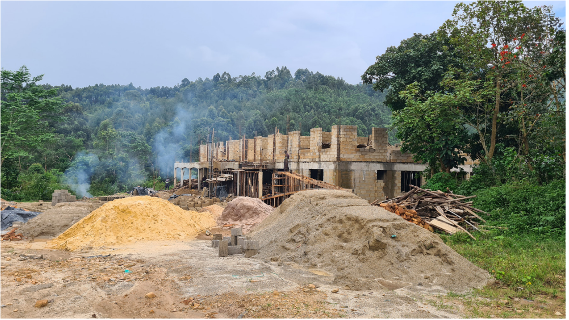
Construction of the new Dental and Vision Clinic at Bwindi Community Hospital is underway! Completion is anticipated by January 2025.
