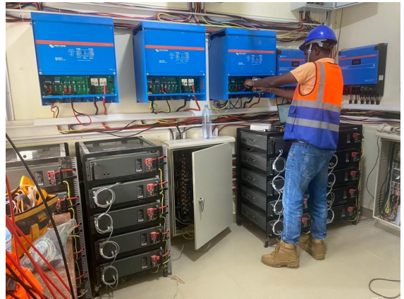
Inside the power auto switch room. This controls the electricity of BCH. This was made possible by Dr Forat and Africomed.
